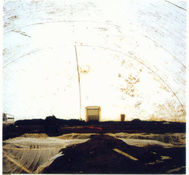
"Inside the air structure, workers labor in comfort and safety. Temperatures hover around 55 degrees regardless of weather outside."
