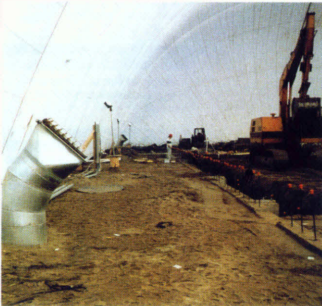
Air is introduced via duct work from 2 heaters. Louver would shut down and retain air if heater malfunctioned, insuring constant balloon pressure.
