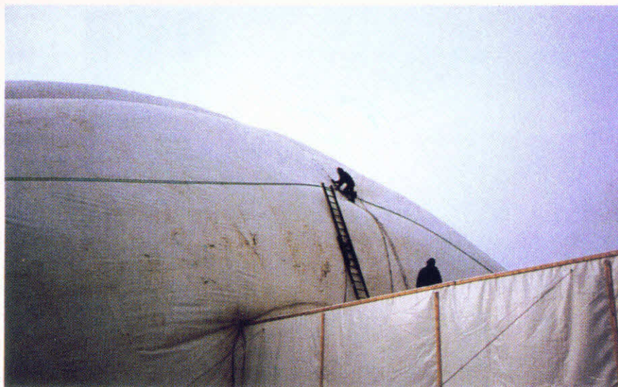
This is pressurization!!!
